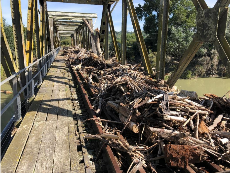
Figure 5 – Debris on the PNGL rail bridge. Image courtesy of HBRC.
