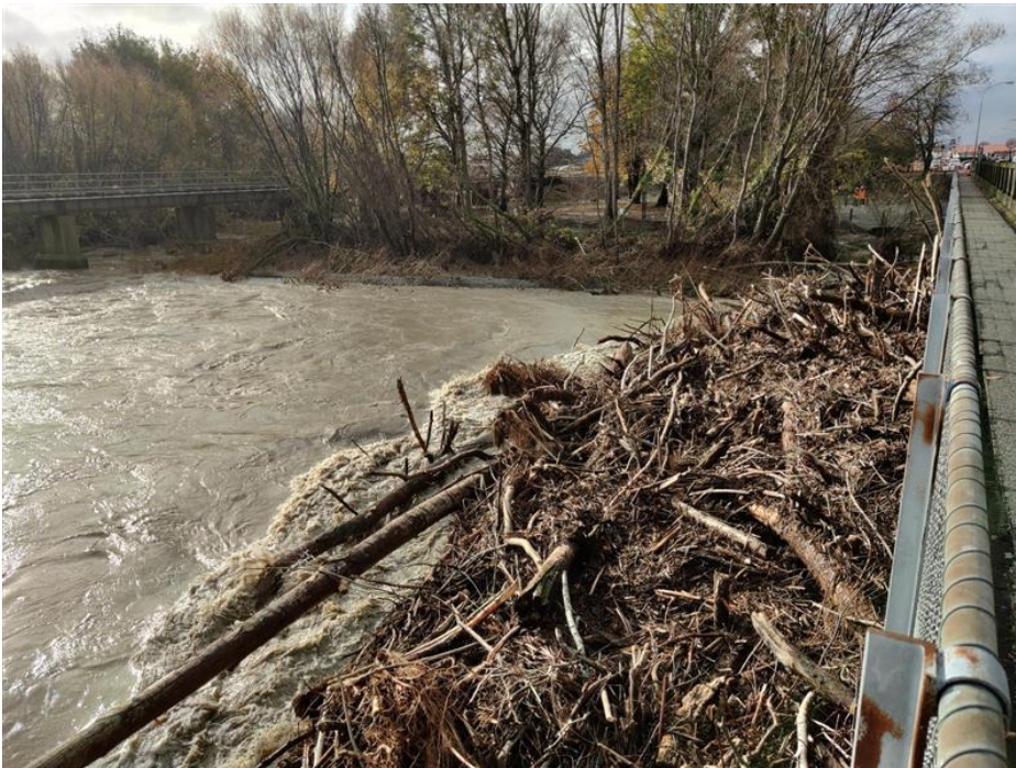
Figure 4 – Debris matt against the Ashburton River Bridge, Canterbury
