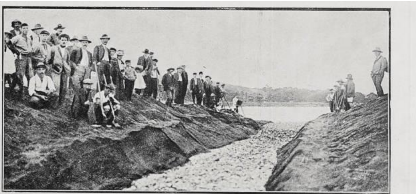
OPENING THE WAIROA BAR, HAWKE'S BAY: THE CHANNEL CUT THROUGH THE SANDSPIT AT THE RIVER MOUTH, AUGUST, 1909. Photos by E. Burridge.
